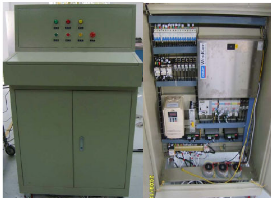
Fig. 8. Control cabinet of small wind turbine
