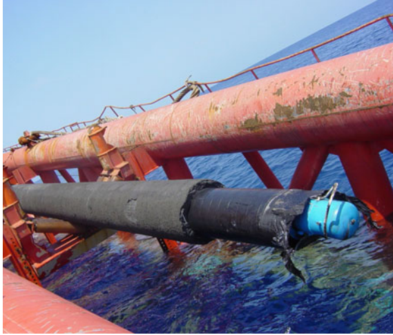
Fig. 3. The ruptured pipe
