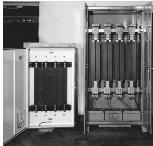
Figure 14.18 Interior view of a high-capacity hybrid power conditioner. (Courtesy of Control Concepts.)
