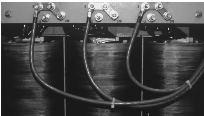
Figure 4.24 A medium-power, three-phase transformer.
