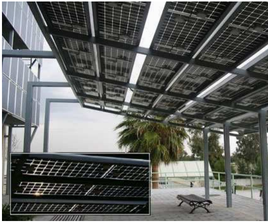
Fig. 8 Photography of “Pergola PV system”
