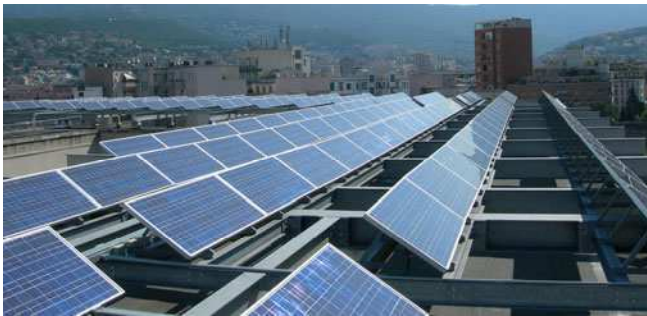
Fig. 3 The GCPV plant installed at the roof top of the Trieste local government building
