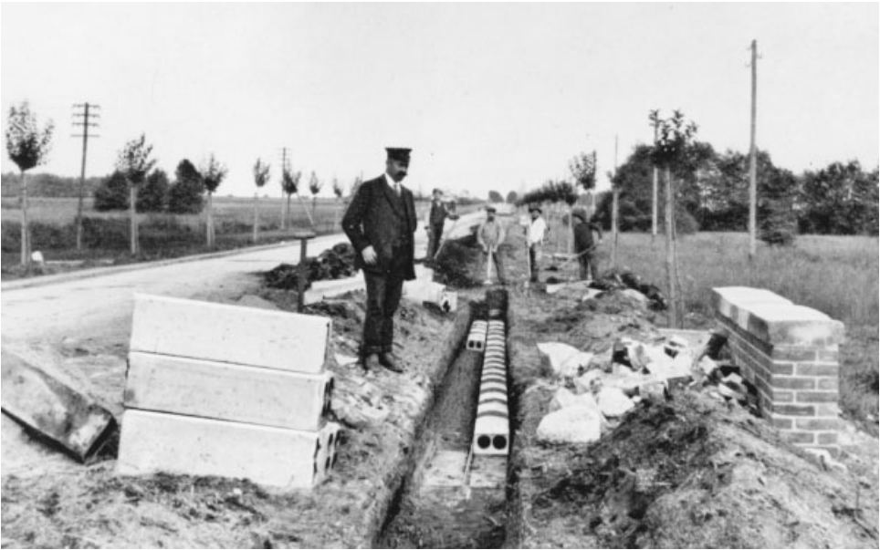
Figure 20.6 Cable duct for Europe's first long-distance telephone cable. (© Siemens-Archiv, Munich.)
