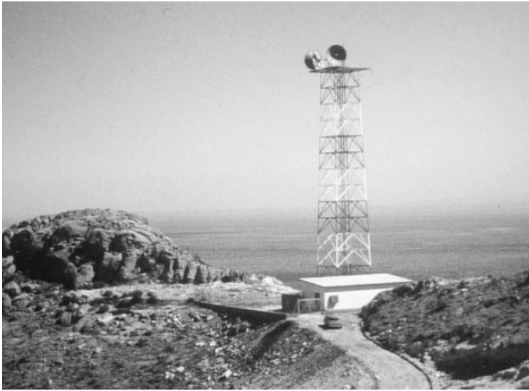
Figure 25.1 Typical radio-relay repeater station in Thailand. (Courtesy of Gerd Lupke.) See insert for a color representation of this figure.
