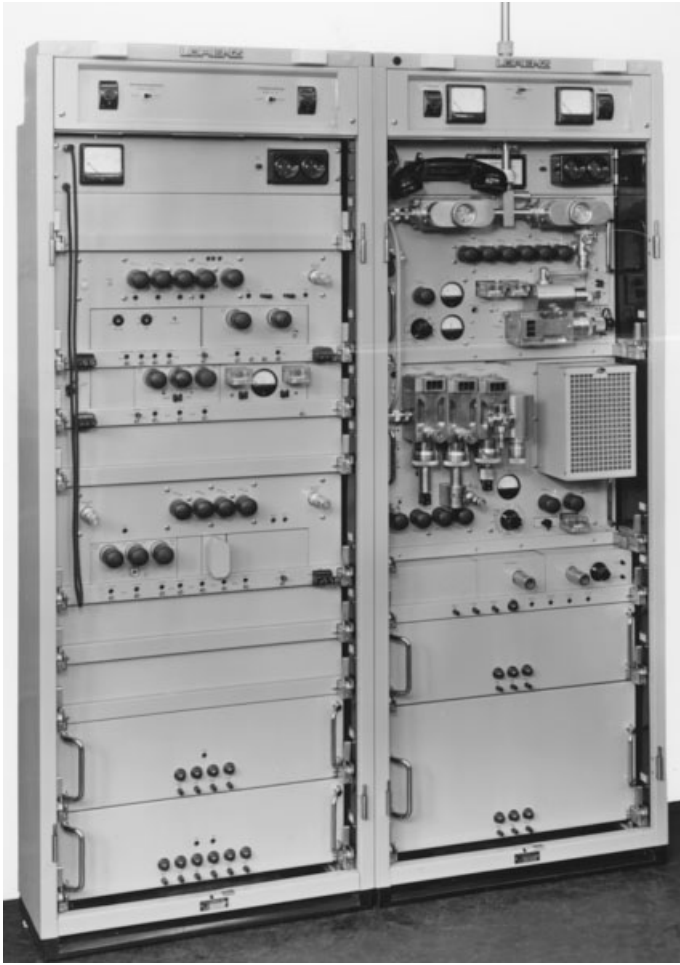
Figure 21.6 Radio-relay terminal with 120-channel 2-GHz equipment, 1955. (Courtesy of Alcatel SEL.)
