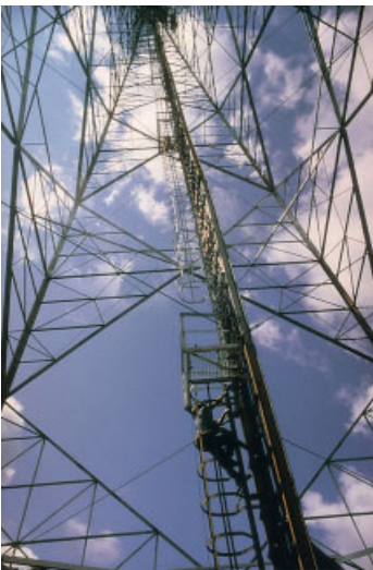
Figure 25.15 Inside view of a self-supporting radio-relay tower in Malaysia, 1975. (Courtesy of Alcatel SEL.)
