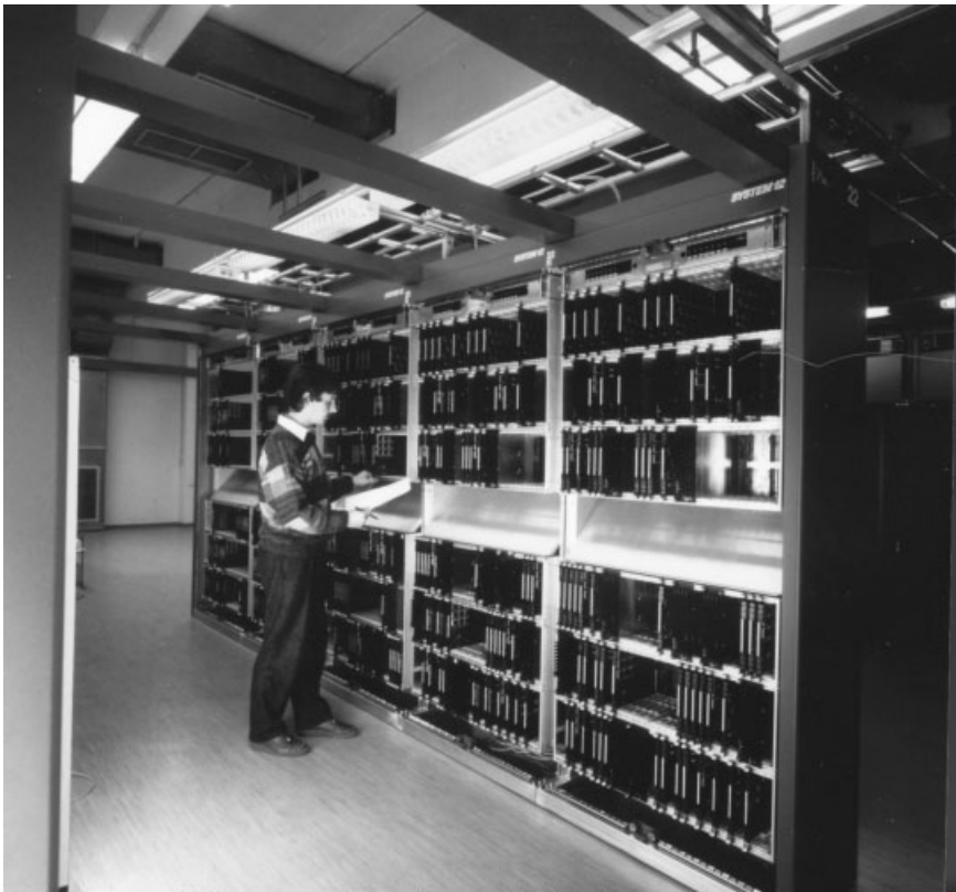
Figure 29.6 System 12 switch installed at Stuttgart, 1982. (Courtesy of Alcatel SEL.)
