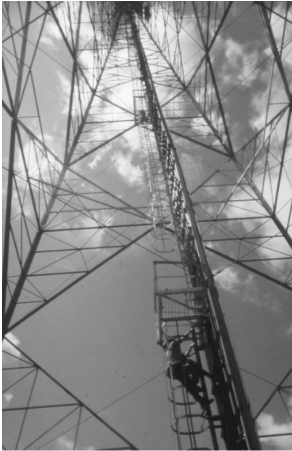
Figure 25.15 Inside view of a self-supporting radio-relay tower in Malaysia, 1975. (Courtesy of Alcatel SEL.) See insert for a color representation of this figure.
