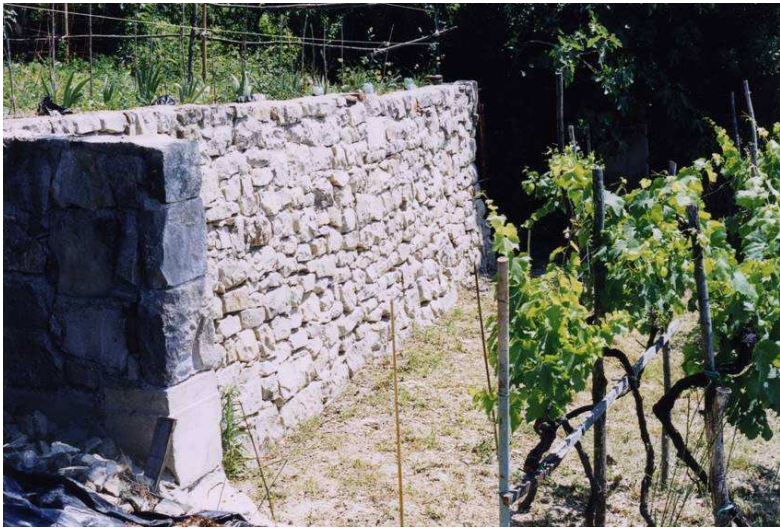
Fig. 10. Rebuilt wall bordering a terraced area near S. Croce, Trieste municipality (source: Antonini M.)
