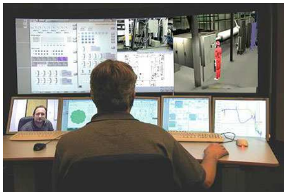
Fig. 2.19 The “cockpit control room” implemented in HAMMLAB for the Extended Teamwork experiment
