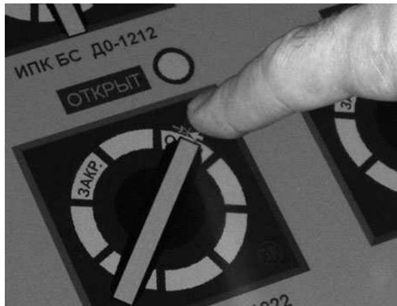
Fig. 8.9 Conventional instrumentation represented using a flat touch screen at the Leningrad Nuclear Power Plant Validation Facility
