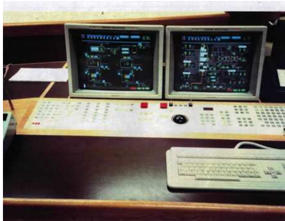
Fig. 8.5 Fully computerised interface in a 1990s gas power plant
